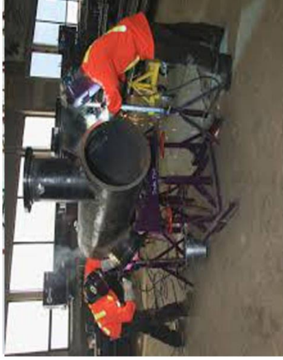
Pipe Fitter work in Jizan JRTP (TR-10) Naseer Saeed Al-Hajri & Partners Company-2017 & 2018
