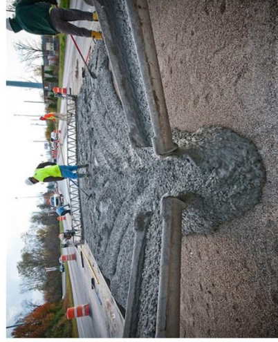
Concrete Pouring 3rd Industrial City Dammam K.S.A. Kanooz Cont. Co. Ongoing Project-2018
